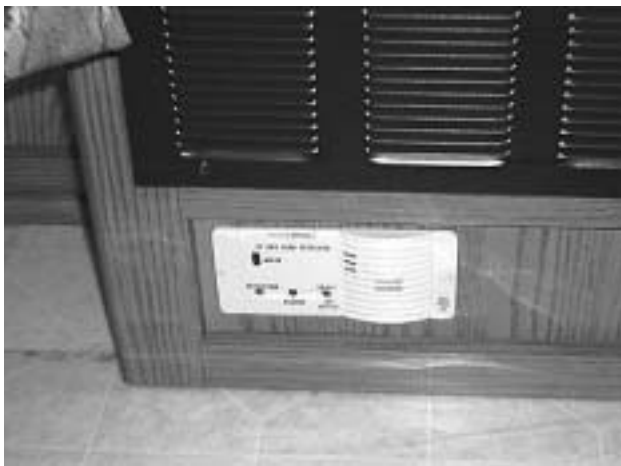
LP Gas Leak Detector
