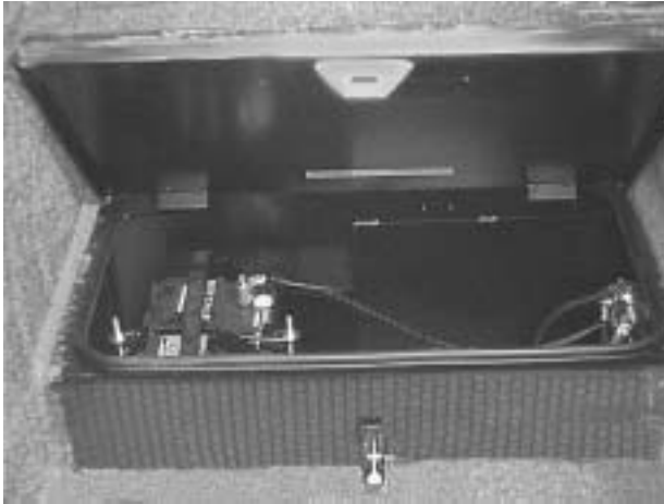
House Battery Storage in Entrance Step Models 27', 29' & 31'
