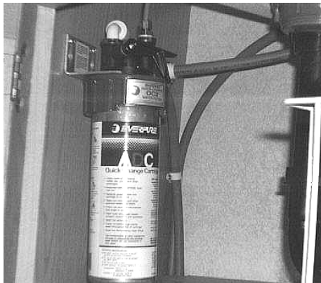
Water Filter Assembly - Below Galley Sink
