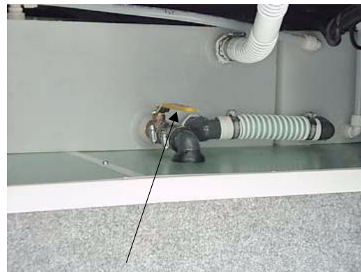
Water Tank Drain Valve in right side compartment toward rear of vehicle
