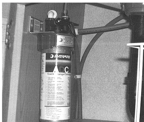
Water Filter Assembly - Below Galley Sink
