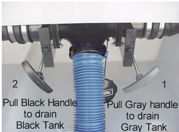
Holding Tank Valves (Typical)
