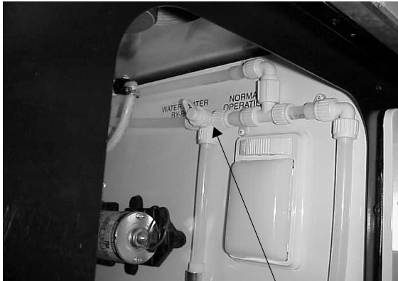
Water Heater Bypass Valve
