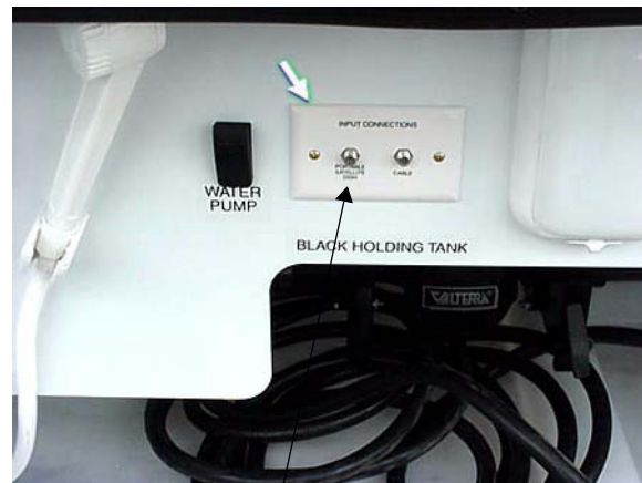
Exterior Connection for Satellite Dishes and Cable TV (In Water Center Compartment)
