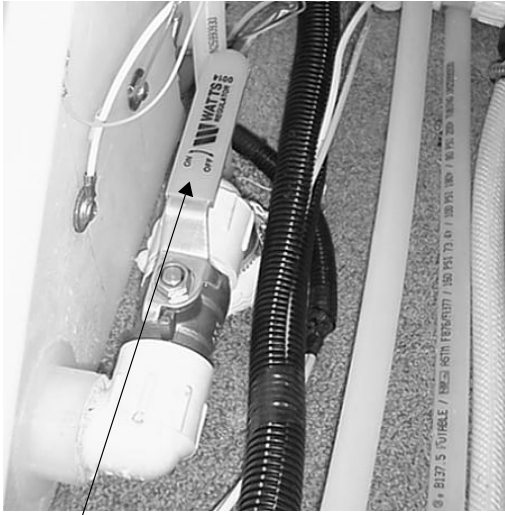
Water Tank Drain Valve (Typical)
