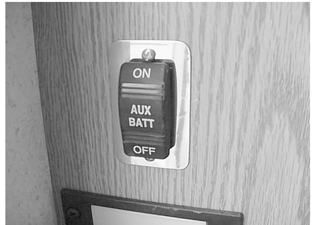
Aux. Batt. Switch (Near entrance door)
