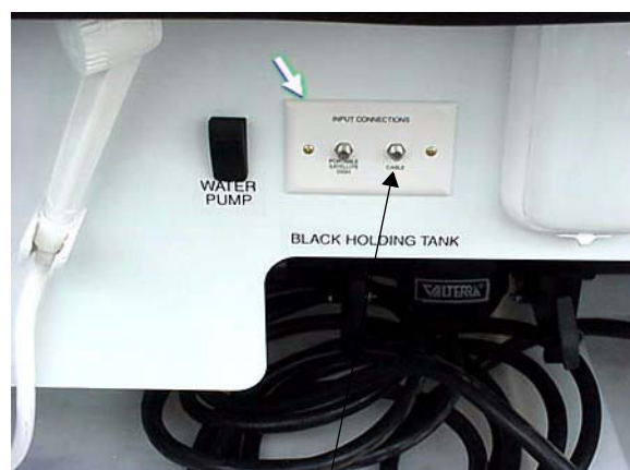
Cable TV Hook-Up in Utility Compartment
