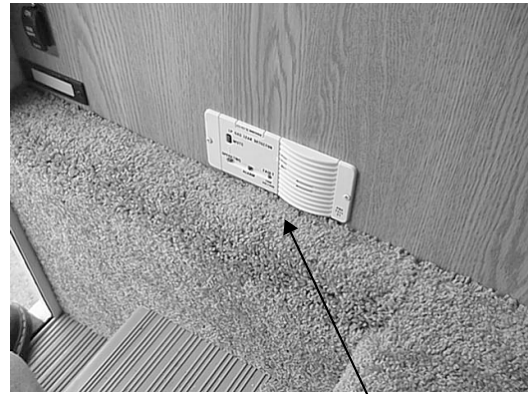
LP Gas Alarm
