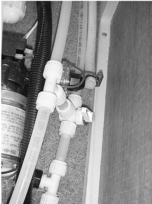
Water Heater By-Pass Valve (Typical) Beneath Bed
