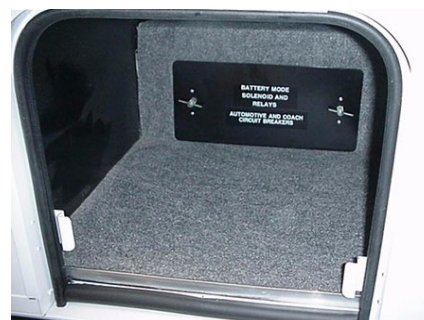
Chassis and House 12V Circuit Breakers behind cover panel in cargo compartment near entrance door
