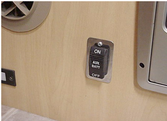
Aux. Batt. Switch (Near entrance door)
