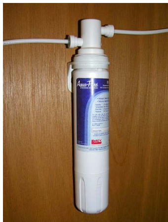
Water Filter Assembly below Galley Sink (Located below galley sink)
