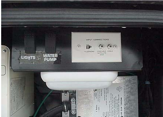
Exterior Input Connections for Satellite Dish, Cable TV and Phone (in Water Center or Shoreline Compartment)
