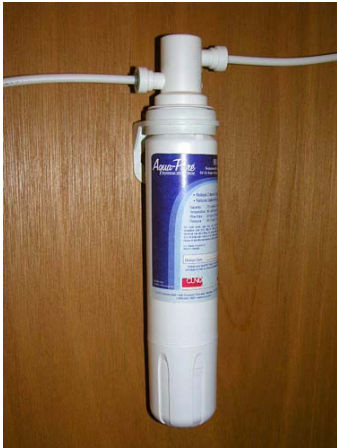
Water Filter Assembly (Located below Galley Sink)
