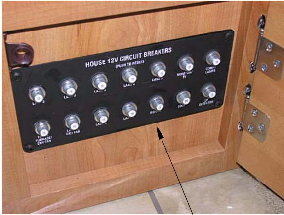
House 12-Volt Circuit Breaker Panel
