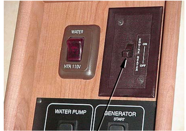
Diesel Engine Heater Switch (typical)
