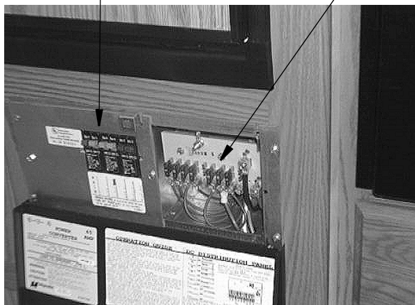
Power Center (Converter)
