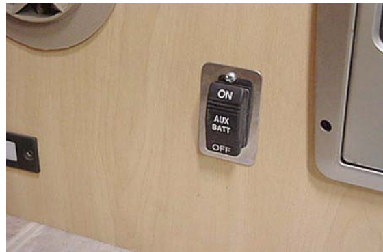
Aux. Batt. Switch - typical (Near entrance door)
