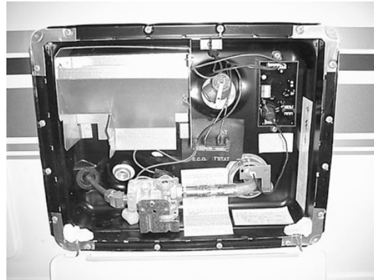
Water Heater Exterior Service Access
