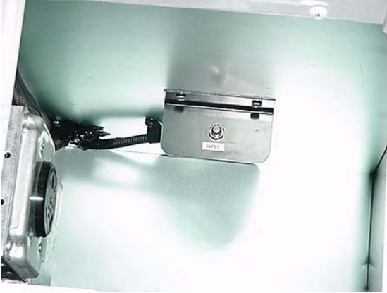
Cable TV Hook-Up in Utility Compartment
