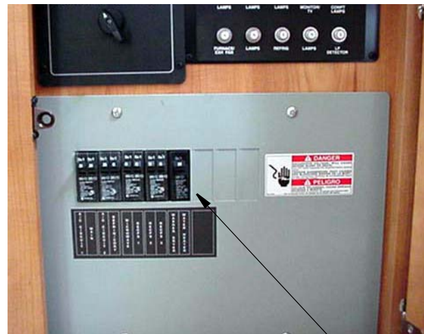
120-Volt House Circuit Breakers
