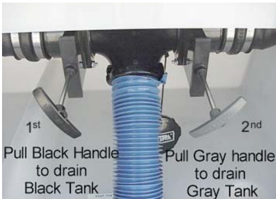
Holding Tank Dump Valves (Typical)
