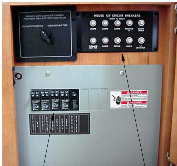
120-Volt House Circuit Breakers
