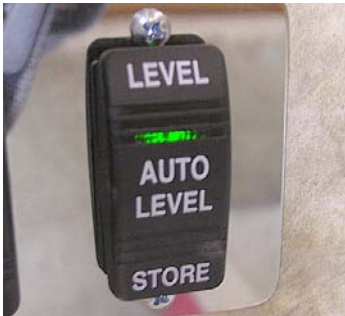
Auto Level Switch inside Entrance Door
