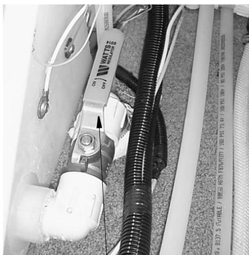
Water Tank Drain Valve (Typical)
