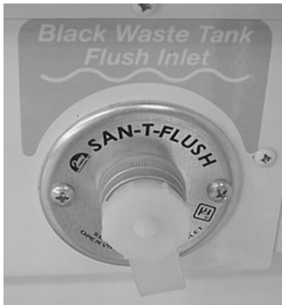
Black Water Tank Flush Inlet (Located in water service center) -Typical View
