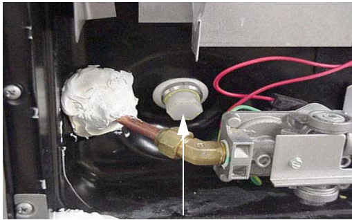
Water Heater Drain Plug (Remove with socket)
