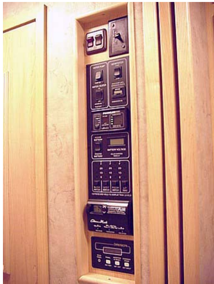
OnePlace Monitor Panel -Typical View
