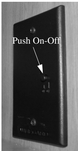
TV Signal Amplifier Power Switch -Typical View
