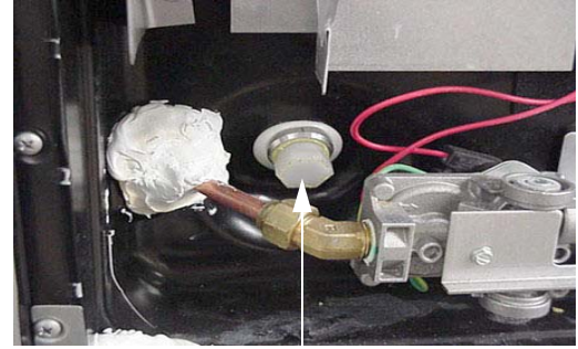
Water Heater Drain Plug (Remove with socket)
