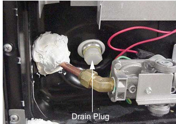
Water Heater Service Access -Typical View
