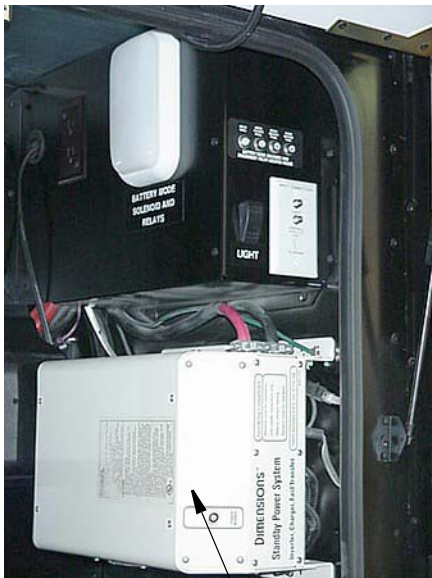
Inverter Charger Unit (Located in utility compartment) -Typical Installation
