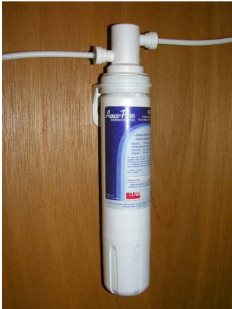
Water Filter Assembly (Located below galley sink)
