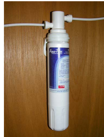
Water Filter Assembly (Located below galley sink)
