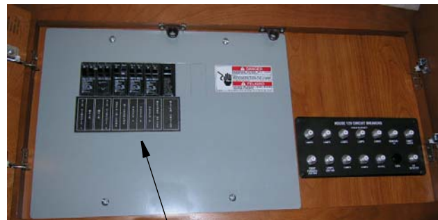
House 120-Volt AC Circuit Breaker Panel
