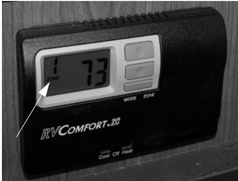
Zone 1 Operation (Living Area/Galley)
