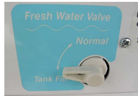
Fresh Water Valve in Tank Fill position (Located in water service center)
