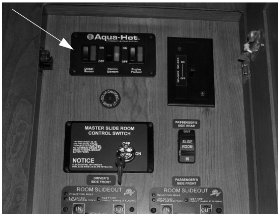
Hydronic Heating System Interior Control Switches (Located near monitor panel) -Typical View
