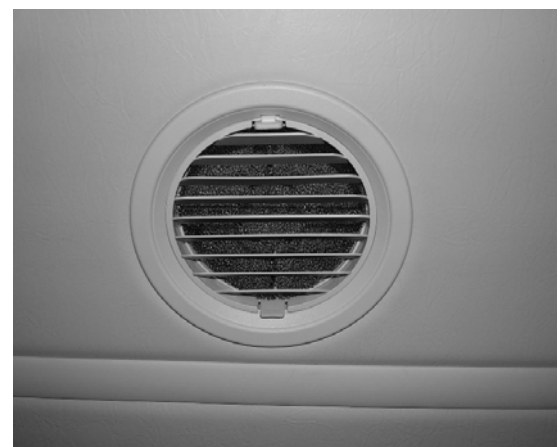
Return Air Vent (Shown with filter installed)
