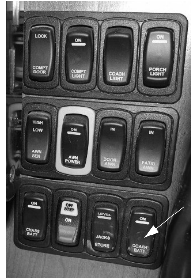
House/Coach Battery Disconnect Switch (Located near entrance door) -Typical View
