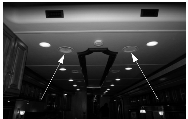
Supply/Return Air Vents (Located throughout the ceiling of the coach) * View looking to rear of coach
