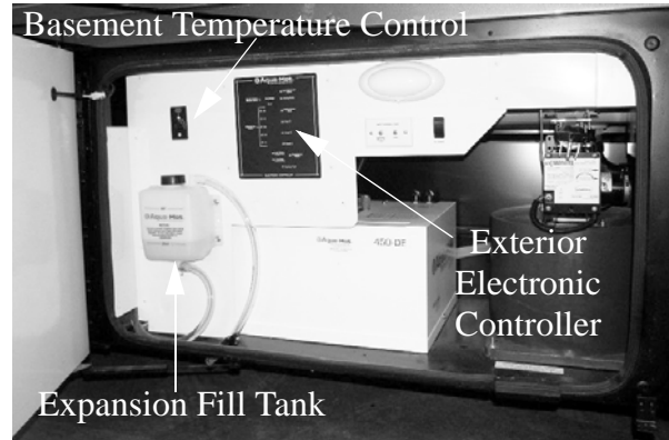
Hydronic Heating System (Located in driver side compartment behind front wheel well) -Typical View
