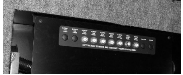
Automotive Chassis and House 12-Volt Circuit Breakers (Located inside passenger compartment) -Typical View
