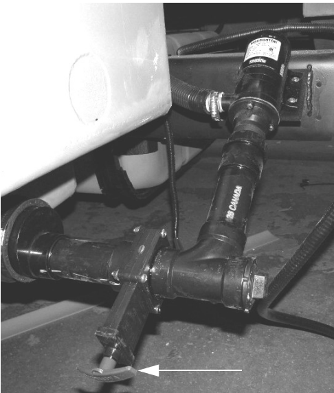
Gray Waste Tank Drain Valve (Located beneath driver side of coach ahead of rear wheel) -Typical View
