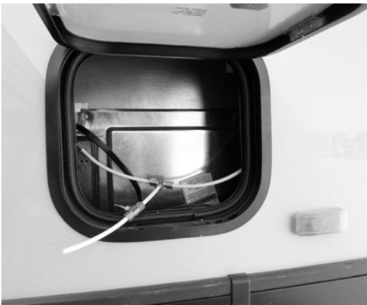
Ice Maker Drain Line (Located in exterior Residential Refrigerator service compartment)
