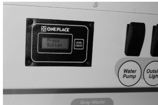
Exterior Monitor Panel (Located in water service center)
