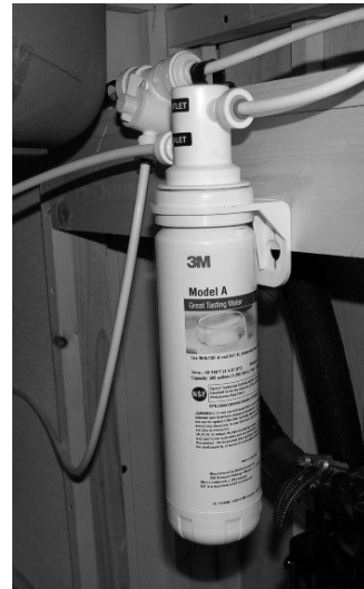
Water Filter Assembly (Located below galley sink) -Typical View
