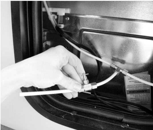
Ice Maker Winterization Drain Valve (Located in exterior Residential Refrigerator service compartment)
