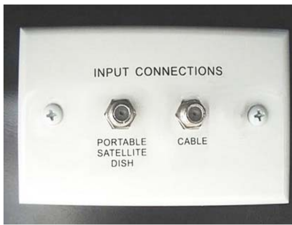
Exterior Connection for Satellite Dish and Cable TV (Located in the shoreline compartment)
