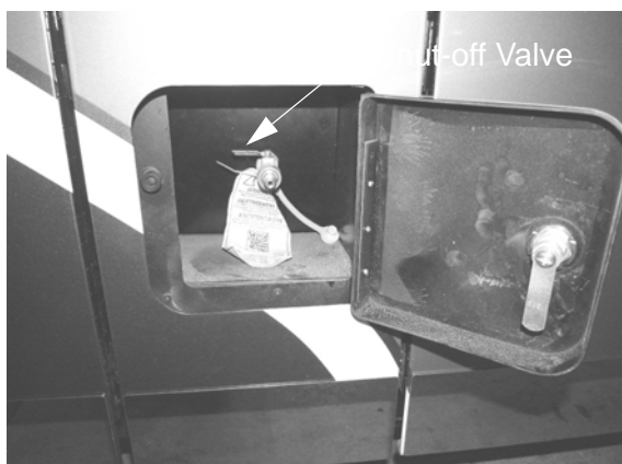
LP Accessory Connection (Located behind lockable access door on passenger side of coach -Typical View
