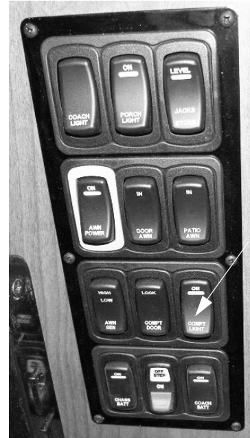
Compartment Lights Switch (Located near entrance door) -Typical View
