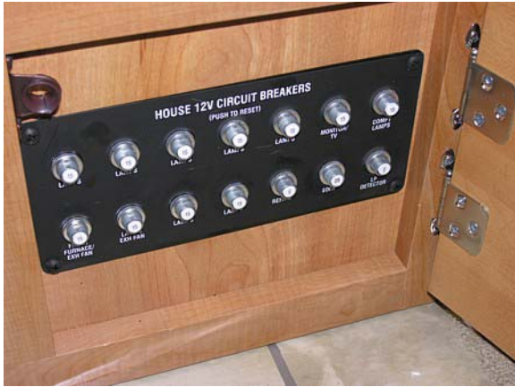
House Circuit Breakers -Typical View
