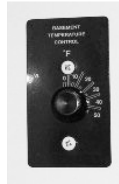
Basement Temperature Control
