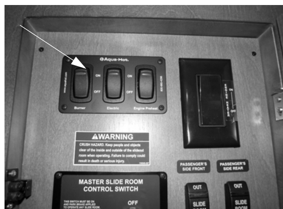
Hydronic Heating System Interior Control Switches (Located near monitor panel) -Typical View
