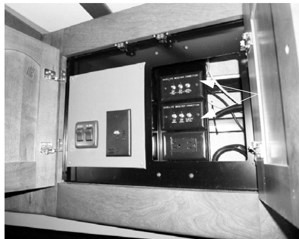
Interior Connections for Satellite Dish (Located in the overhead compartment above entrance door)
