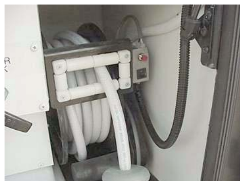
Water Hose Reel (Located in the water service center) -Typical installation shown
