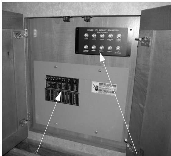
120-Volt House Circuit Breakers
