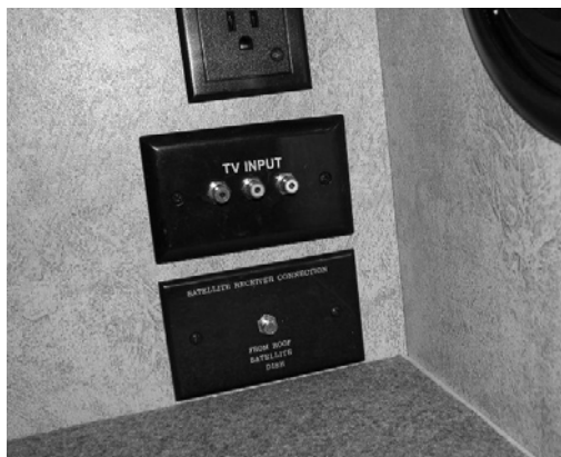
Bedroom DVD/Satellite Receiver Connection -Typical View
