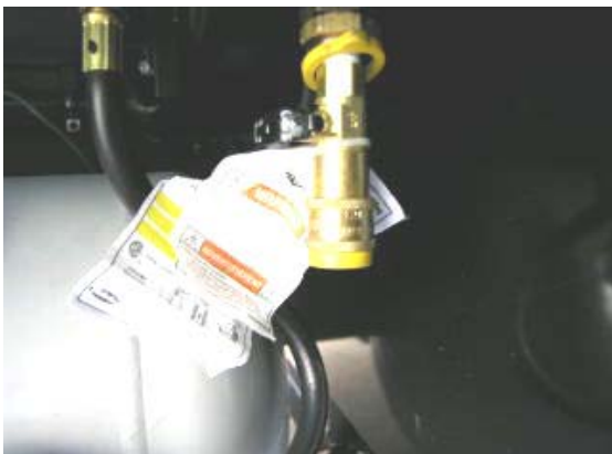
LP Accessory Connection (Located behind LP Tank access door on passenger side of coach) -Typical View
