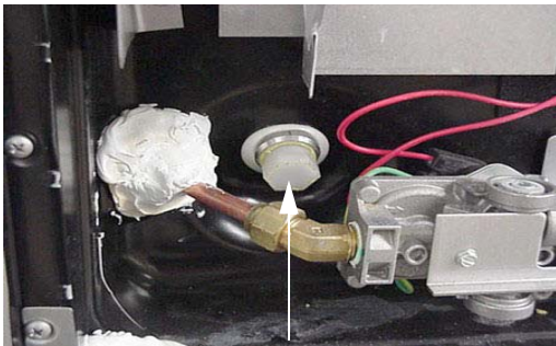
Water Heater Drain Plug (Remove with socket)
