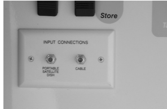
Exterior Connections for Cable TV and Satellite Dish (Located in water service center) -Typical View
