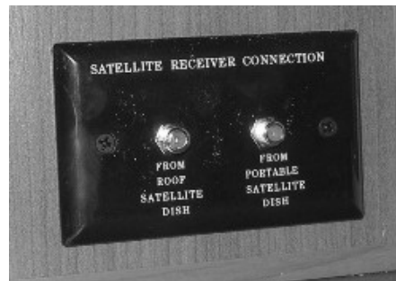
Interior Connection for Satellite Dish (Located in cabinet near TV) -Typical View
