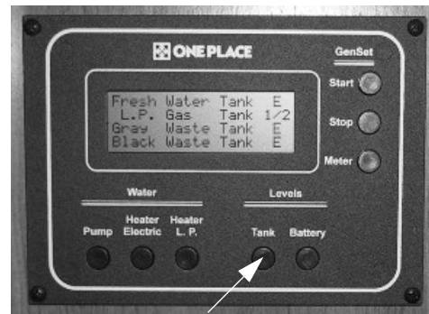
Tank Levels Switch
