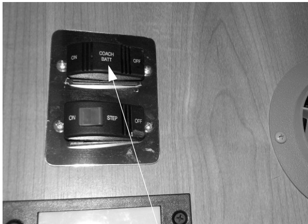
House/Coach Battery Disconnect Switch (Located on galley end) -Typical View
