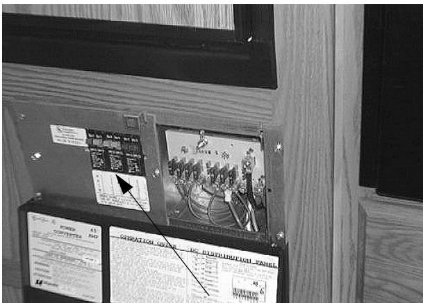
120-Volt House Circuit Breakers -Typical View
