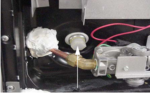
Water Heater Drain Plug (Remove with socket)
