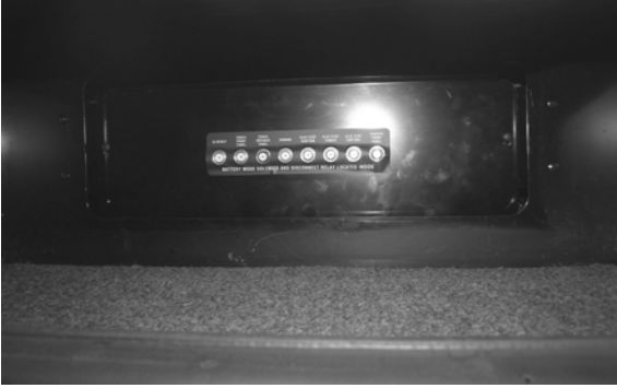
Automotive Chassis and House 12-Volt Circuit Breakers (Located inside passenger compartment) -Typical View
