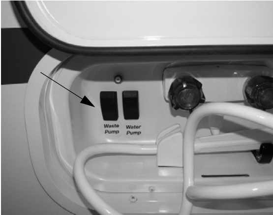
Waste Pump Switch (Located near exterior shower) -Typical View
