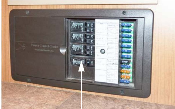
120-Volt Circuit Breakers -Typical View
