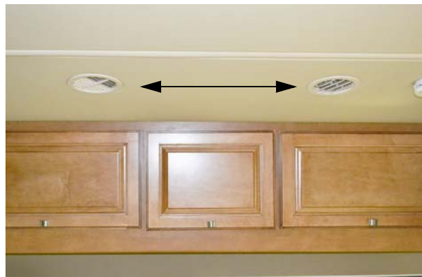
Supply/Return Air Vents (Located throughout the ceiling of the coach) -Typical View
