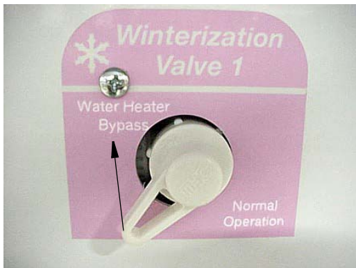
Winterization Valve 1 (See the “Water System Drain Valve Locations” chart at the end of this section for location on your coach)
