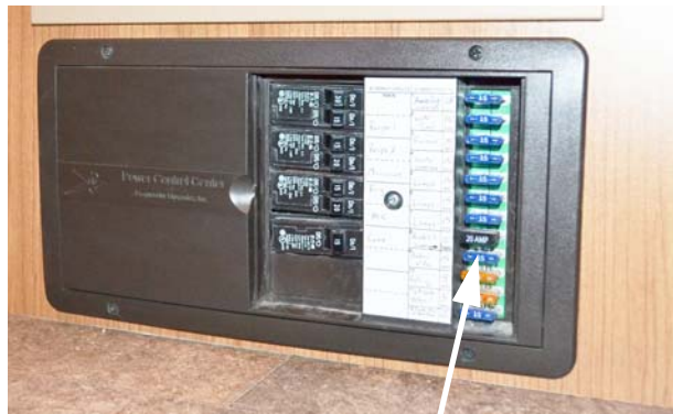
House 12-Volt Fuses (Located on the right-hand side of the Power Converter) (Models 27N and 30T) -Typical View
