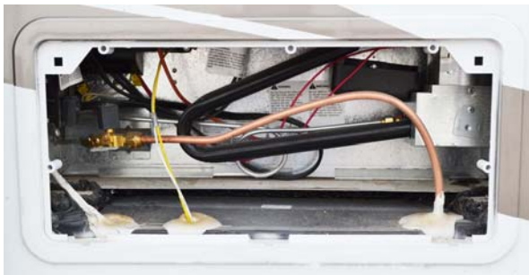
Refrigerator Access Compartment -Typical View
