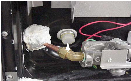
Water Heater Drain Plug (Remove with socket)
