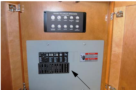
120-Volt House Circuit Breakers -Typical View
