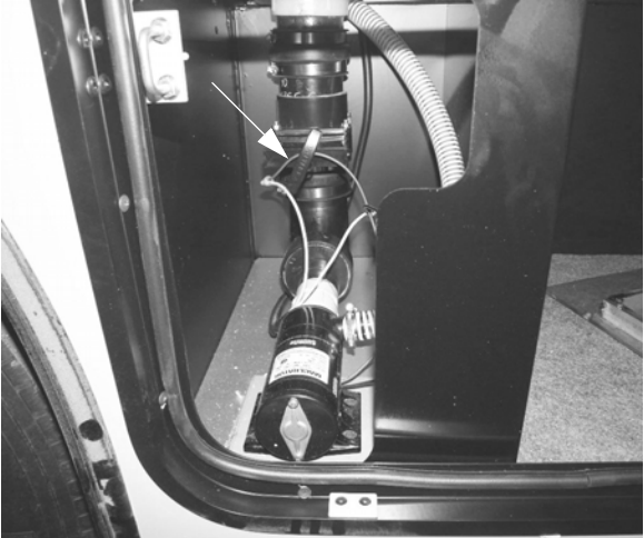
Black Waste Tank Drain Valve #1 (Front) (Located in passenger side compartment ahead of rear axle) -Typical View
