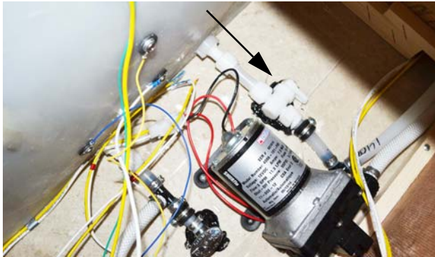
Waterline Drain Valve -Typical View
