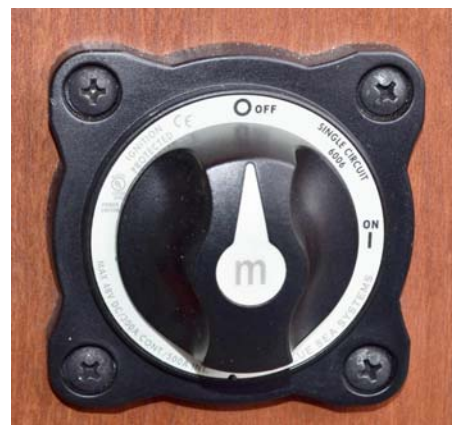
House/Coach Battery Disconnect Switch (Located near entrance door) -Typical View
