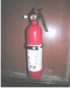
Fire Extinguisher (Typical installation - your coach may vary according to model and floorplan)
