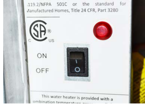
Water Heater (Tankless) Power Switch
