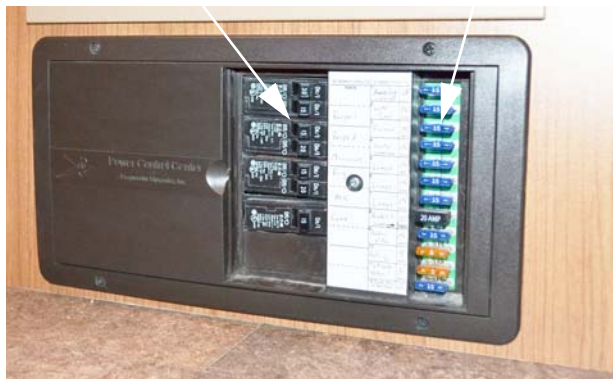
Power Center (Converter) -Typical View
