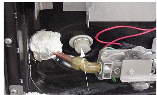
Water Heater Drain Plug (Remove with socket)
