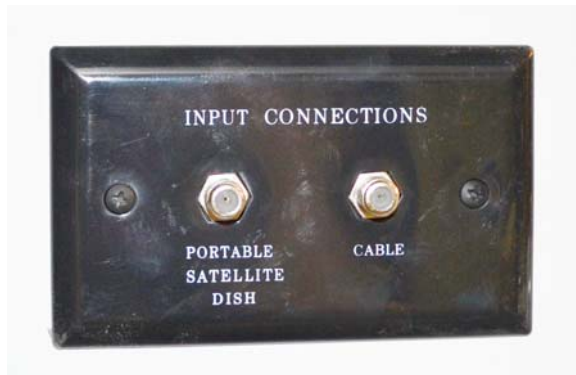
Exterior Cable TV and Satellite Connections (Located in shoreline or utility compartment, depending on model)
