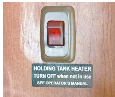
Holding Tank Heater Switch -Typical installation shown
