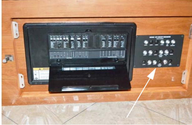
House Circuit Breakers -Typical View
