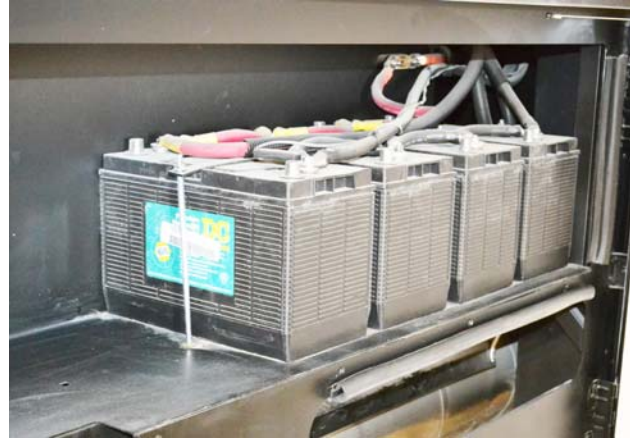
House/Coach Batteries -Typical View
