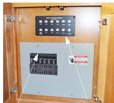
120-Volt House Circuit Breakers
