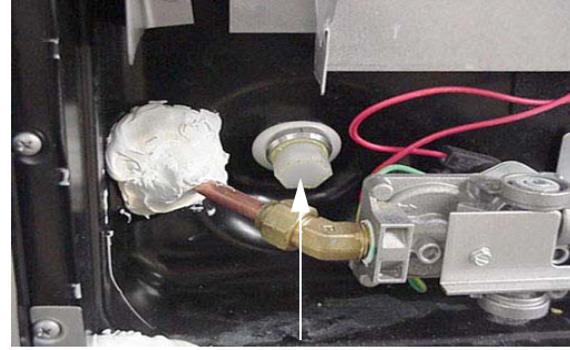
Water Heater Drain Plug (Remove with socket)
