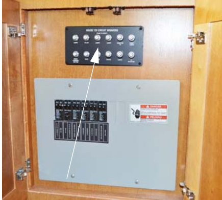
House 12V Breakers -Typical View
