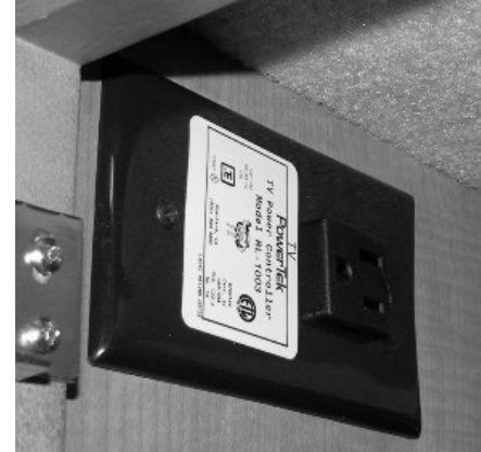
Front TV Ignition Switch Interlock -Typical View
