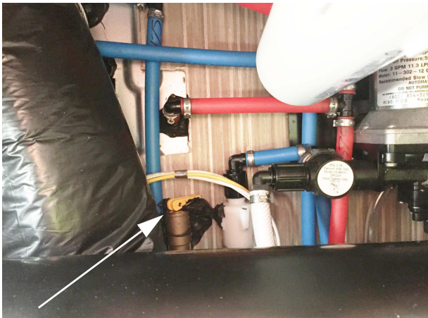
Water Heater Drain (Yellow) Valve
