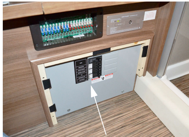
120-Volt Circuit Breakers -Typical View
