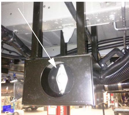
Waste Pump (Located beneath motorhome)
