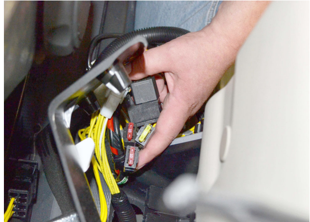
Trailer Plug and Step Fuses (Located behind plastic panel on pillar behind passenger seat)
