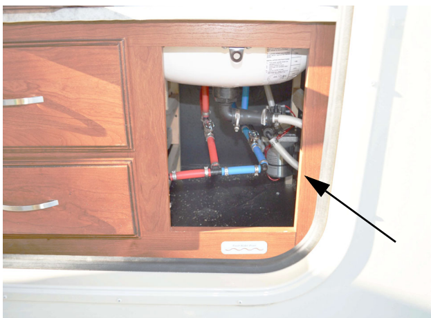
Exterior Sink Pump (Located in the passenger side compartment behind rear axle) -Typical View
