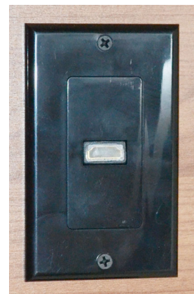
HDMI Connection (Located in a cabinet near TV) -Typical View
