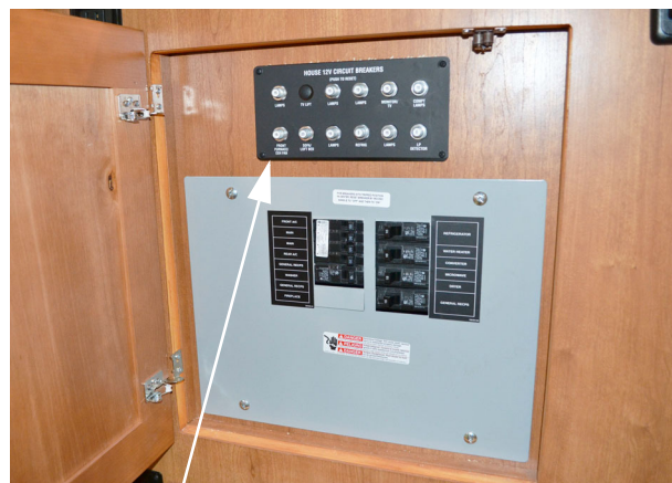
House 12-Volt Circuit Breakers
