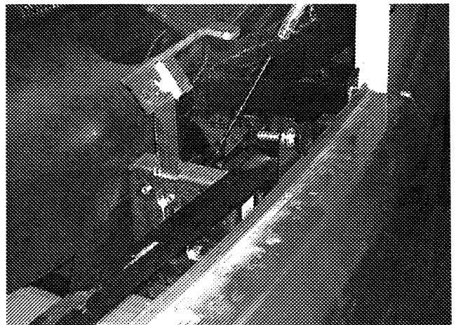
Generator Service Latch - Unlocked
