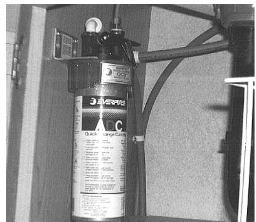
Water Filter Assembly - Below Galley Sink
