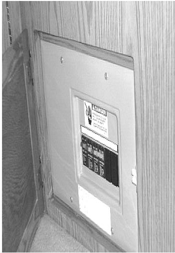
House 110-volt Breaker Panel
