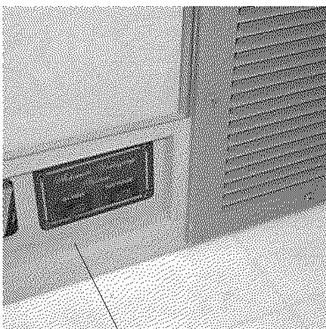
Automatic Winterization Panel
