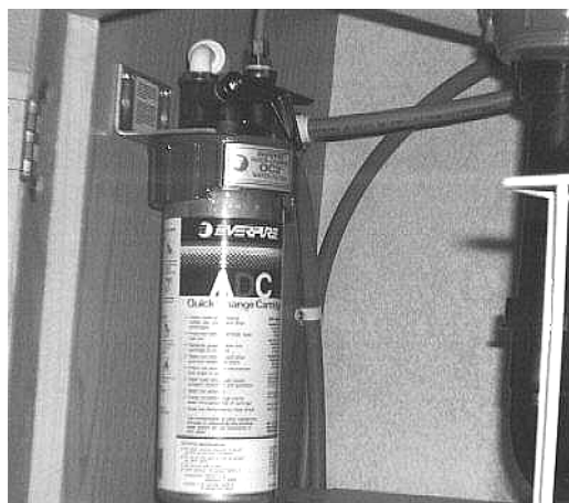
Water Filter Assembly - Below Galley Sink
