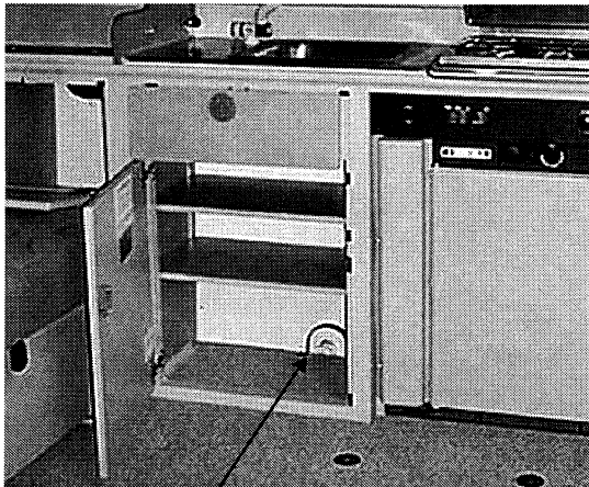
Water Line Drain Valve
