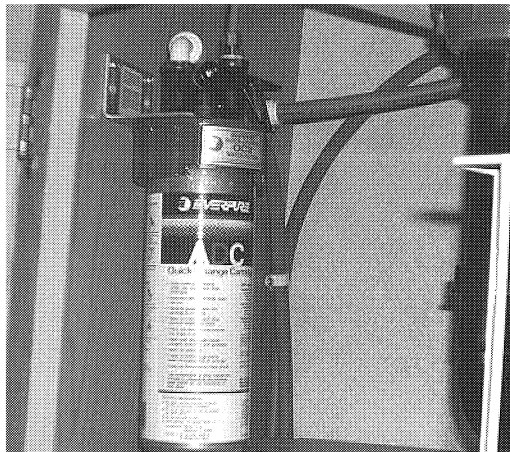
Water Filter Assembly - Below Galley Sink
