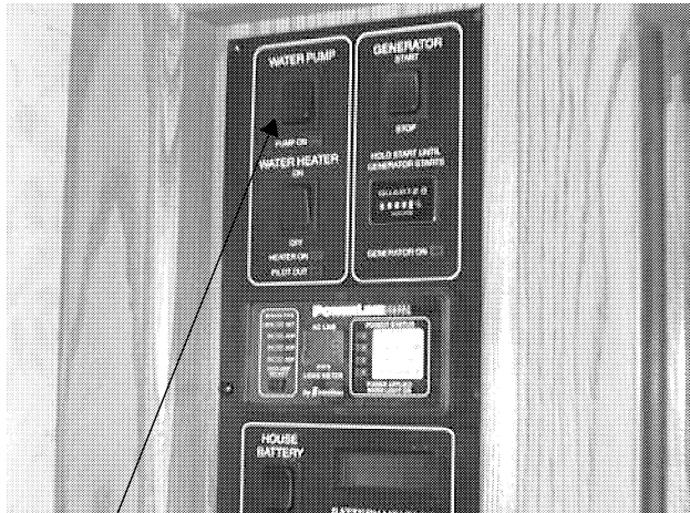
Water Pump Switch
