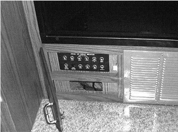
House 12V Breakers (below refrigerator)
