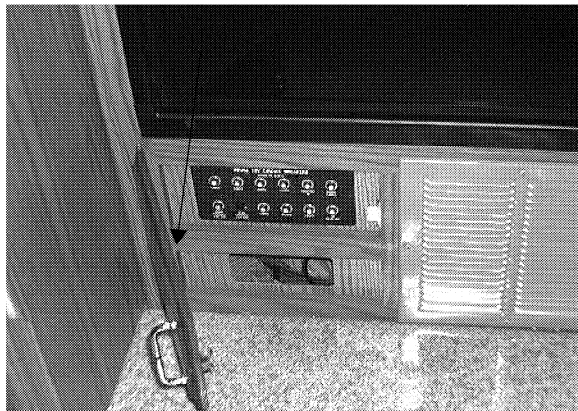
House 12-Volt Circuit Breaker Panel
