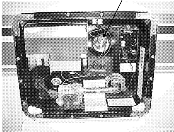
Water Heater Exterior Service Access
