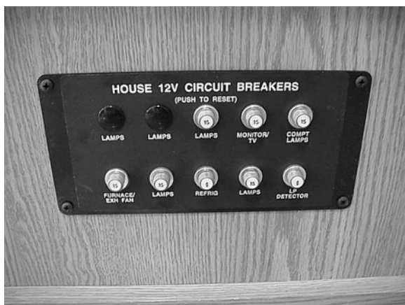
House 12V Circuit Breakers
