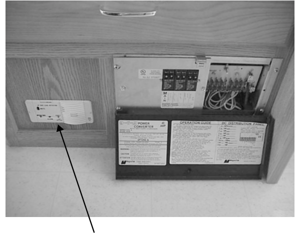
LP Gas Alarm
