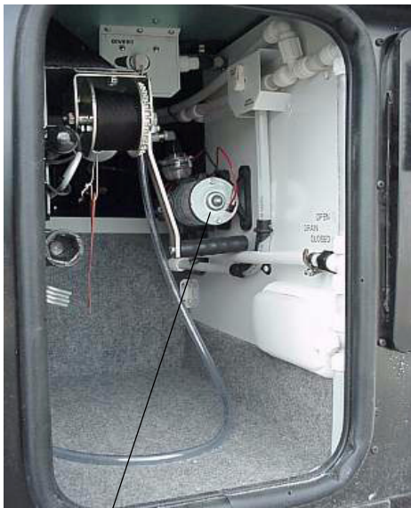
Water Pump in right front compartment
