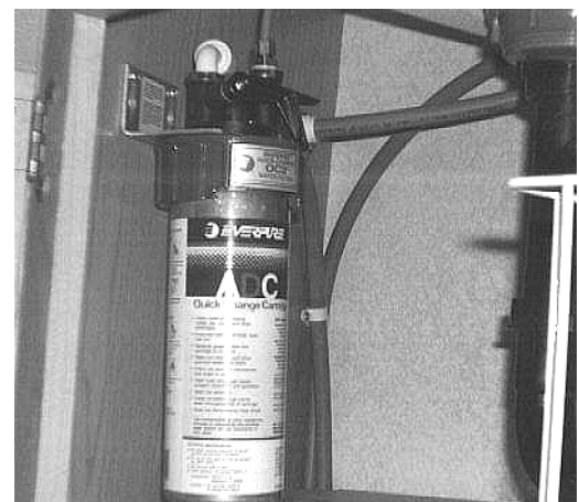
Water Filter Assembly - Below Galley Sink
