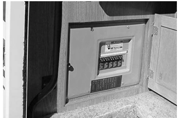
110-Volt Circuit Breaker Panel
