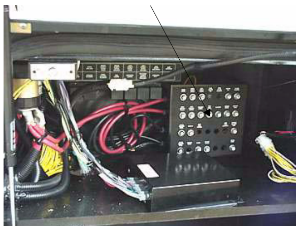
Automotive/Chassis Electrical Center (Left Front Compartment)
