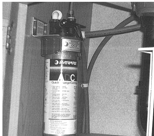
Water Filter Assembly - Below Galley Sink
