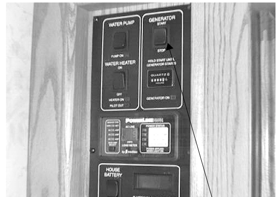
Generator Switch and Hourmeter
