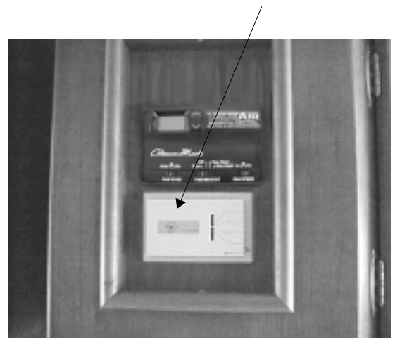
Power Ventilator Thermostat - Galley
