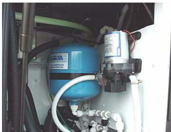
Water Line Drain Valves (in water pump compartment)
