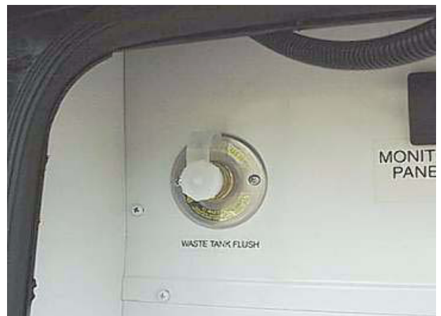
Black Tank Flush Inlet
