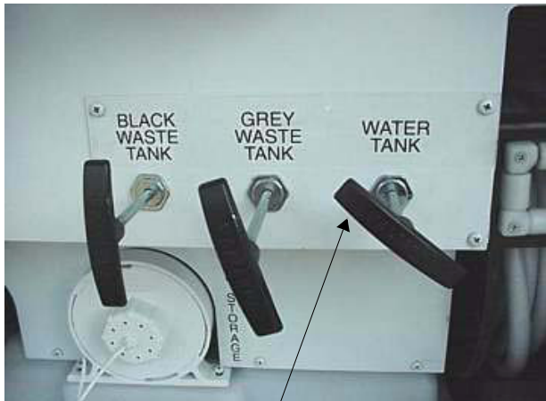
Water Tank Drain Valve (pull to open)
