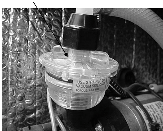
Water Pump Strainer
