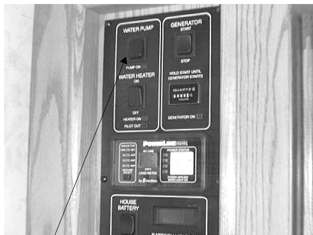
Water Pump Switch
