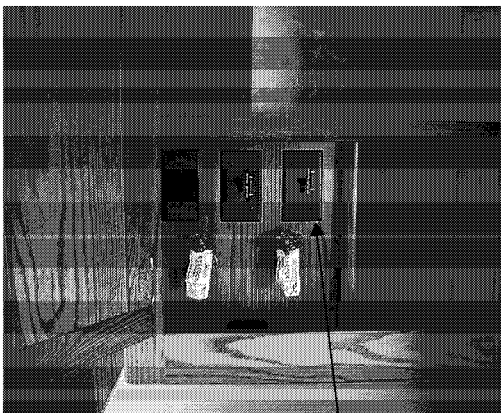
Engine Block Heater Switch (Typical)
