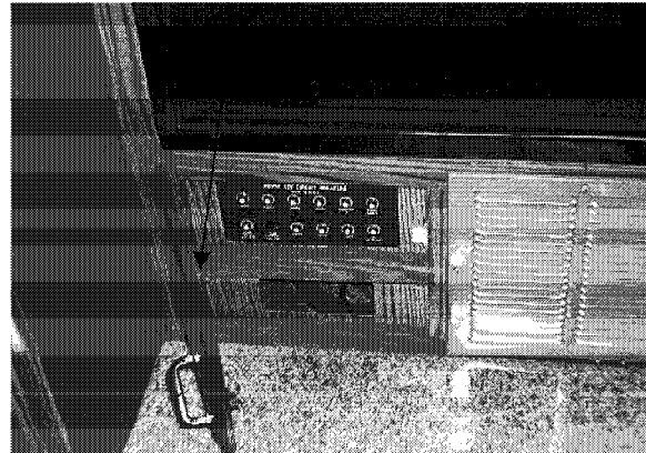
House 12-Volt Circuit Breaker Panel
