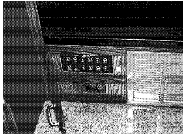
House 12V Breakers (below refrigerator)
