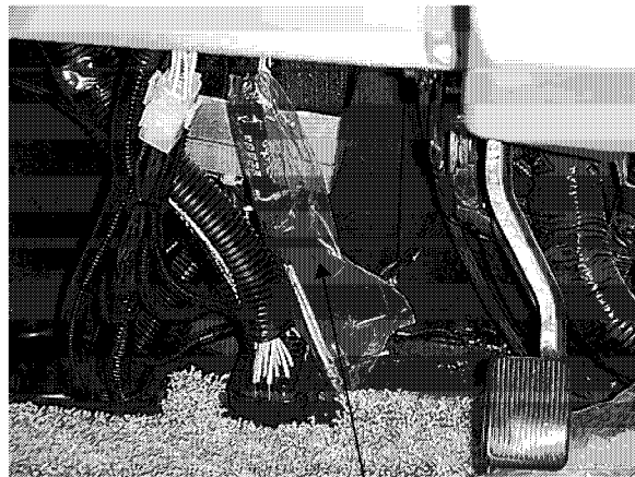
CB Wires (in plastic sheath)
