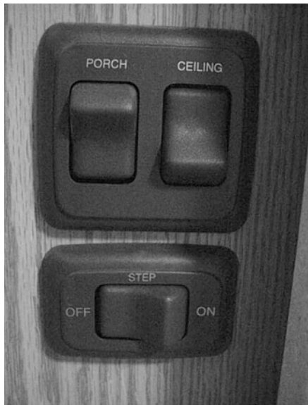
Entry Switch Panel
