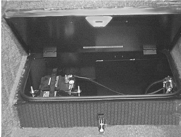
House Battery Storage in Entrance Step Models 24F, & 24V, 27L, 29B & 31C/T
