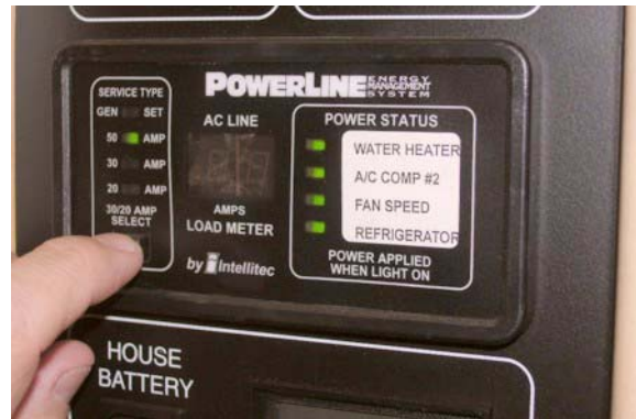
PowerLine EMS Display on Monitor Panel - typical
