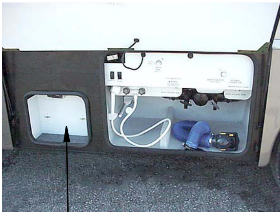
Water drain valves located behind access panel
