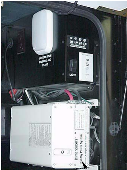
Inverter Charger Unit Location in utility compartment
