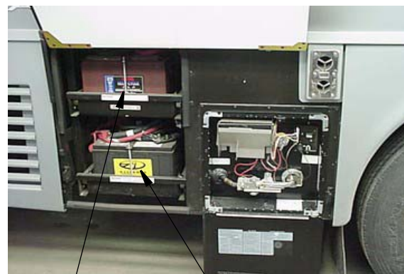
House Batteries Chassis Batteries
