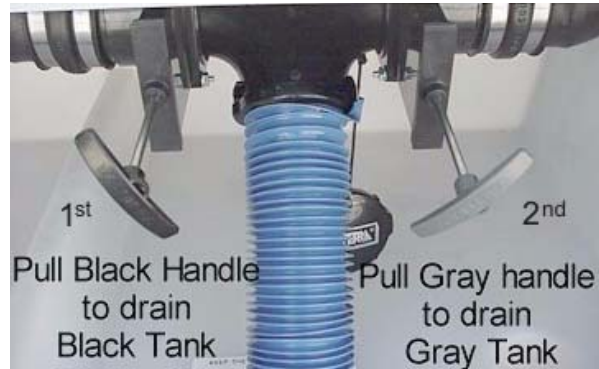
Holding Tank Valves (Typical)
