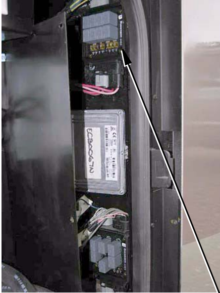
Towing Package fuses are on fuse block
