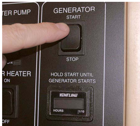
Generator Switch and Hourmeter on monitor panel
