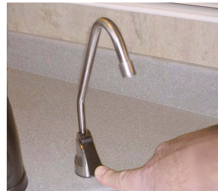
Filtered Water Faucet
