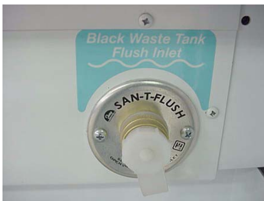
Black Water Tank Flush Inlet in Water Service Center (typical)
