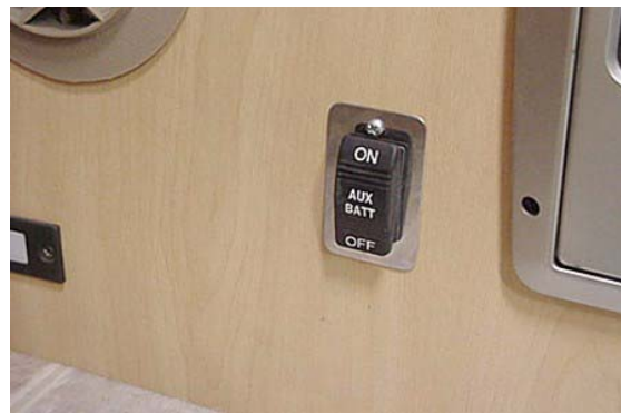
Aux. Batt. Switch - typical (Near entrance door)
