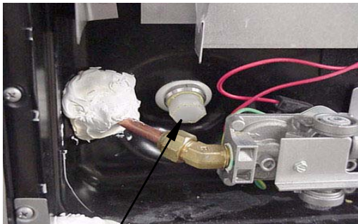
Water Heater Drain Plug Remove with socket.
