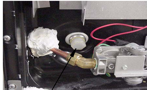
Water Heater Drain Plug Remove with socket.
