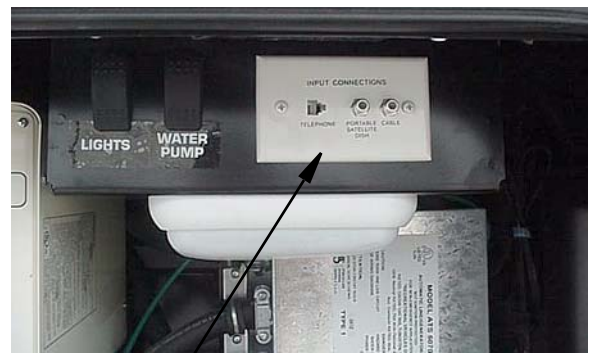
Exterior Input Connections for Satellite Dish, Cable TV and Phone (in Water Center or Utility Compartment)
