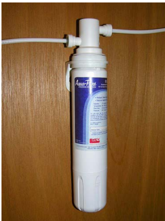
Water Filter Assembly below Galley Sink
