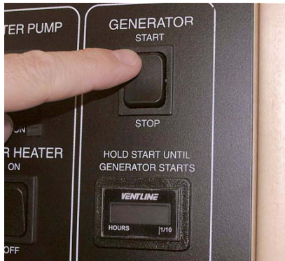
Generator Switch and Hourmeter
