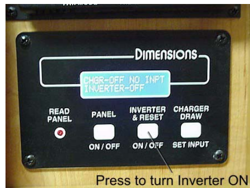
Inverter/Charger Control Panel
