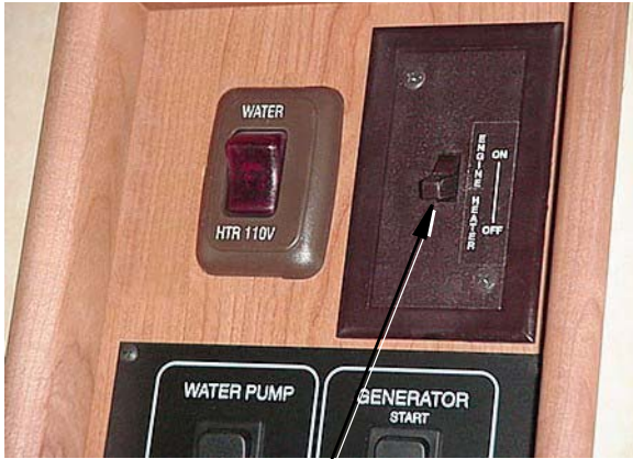
Diesel Engine Heater Switch (Typical)
