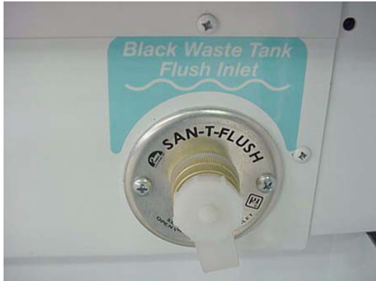
Black Water Tank Flush Inlet in Water Service Center (typical)
