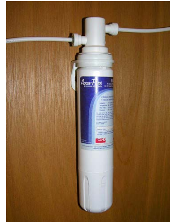
Water Filter Assembly below Galley Sink
