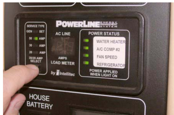
PowerLine EMS Display on Monitor Panel - Typical
