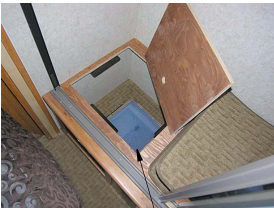
AC/Furnace Filter under wardrobe floor panel
