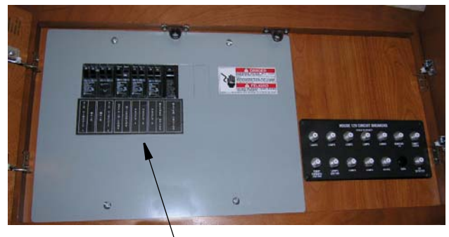
House 120-Volt AC Circuit Breaker Panel
