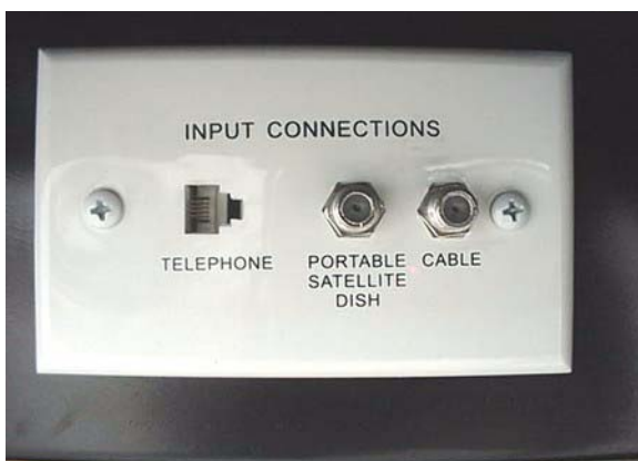
Exterior Connection for Phone, Satellite Dish and Cable TV (In Utility Compartment)
