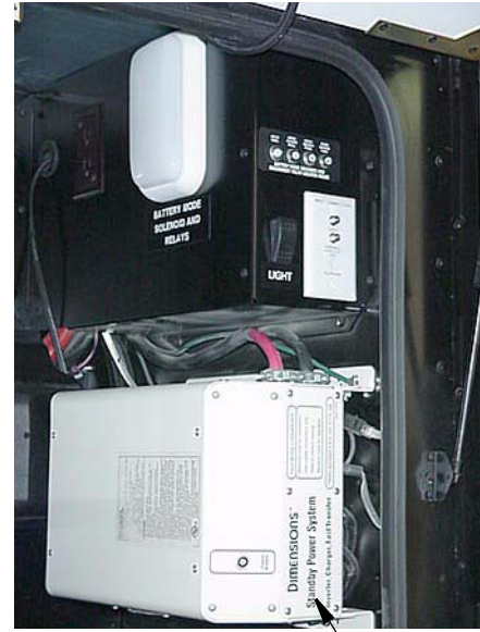
Inverter Charger Unit Location in utility compartment
