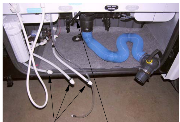
Water Line Drains (remove caps and turn valves to drain lines)
