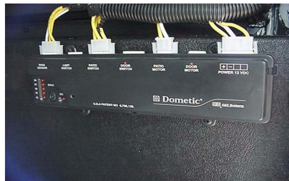
Awning Control Box (located in exterior compartment)
