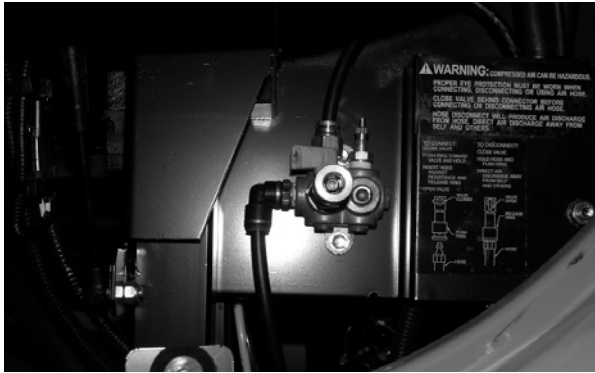
Quick Connect Air Coupler and Air Valve at front end of coach
