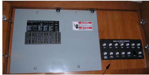
House 12-Volt Circuit Breaker Panel
