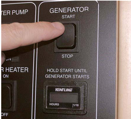
Generator Switch and Hourmeter on monitor panel
