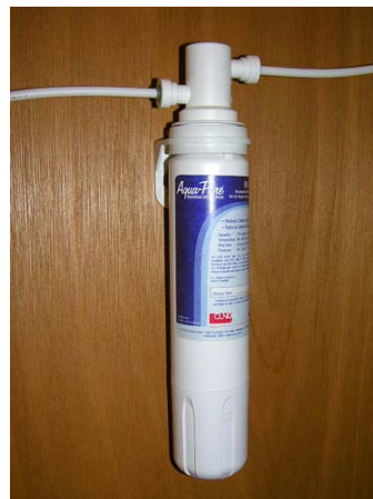
Water Filter Assembly below Galley Sink
