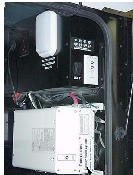
Inverter Charger Unit Location in utility compartment
