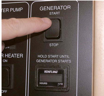
Generator Switch and Hourmeter
