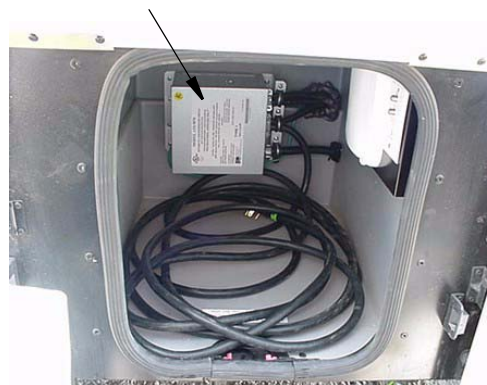
Power Transfer Switch
