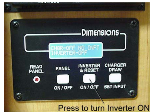
Inverter/Charger Control Panel
