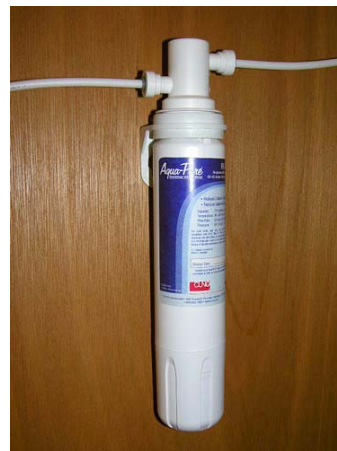
Water Filter Assembly below Galley Sink
