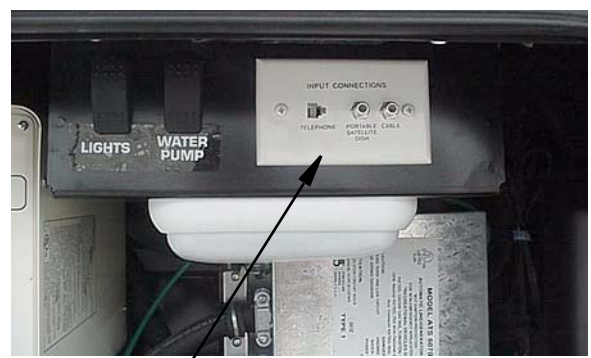
Exterior Input Connections for Satellite Dish, Cable TV and Phone (in Water Center or Utility Compartment)
