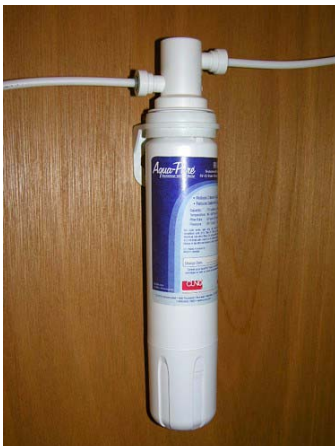
Water Filter Assembly below Galley Sink
