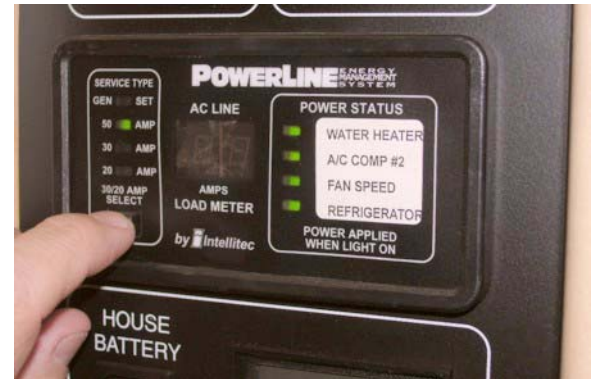
PowerLine EMS Display on Monitor Panel - Typical
