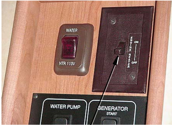
Diesel Engine Heater Switch (Typical)
