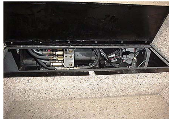
Hydraulic Pump beneath Entry Step
