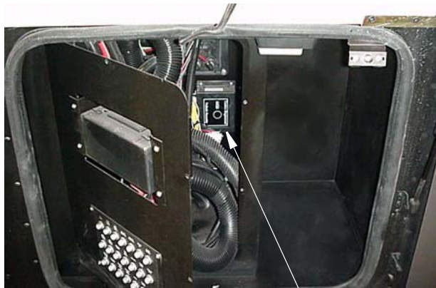
Keyless Entry Control Box in 12-volt electrical compartment.
