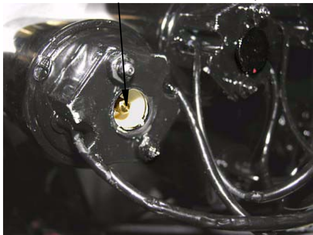
Hydraulic Pump Solenoid Valve
