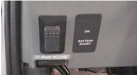
Battery Boost Switch
