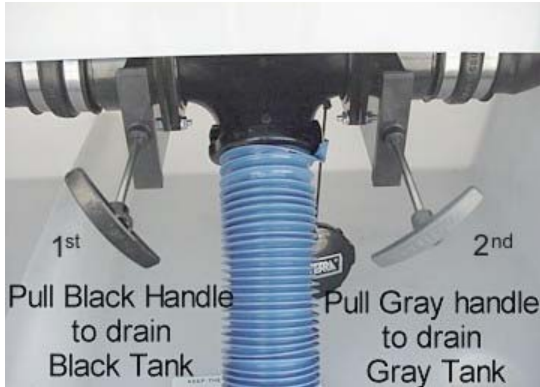
Holding Tank Dump Valves (Typical)
