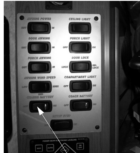
Chassis Battery Disconnect Switch (located inside the entrance door)
