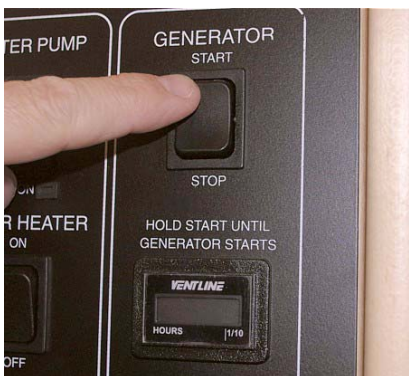
Generator Switch and Hourmeter
