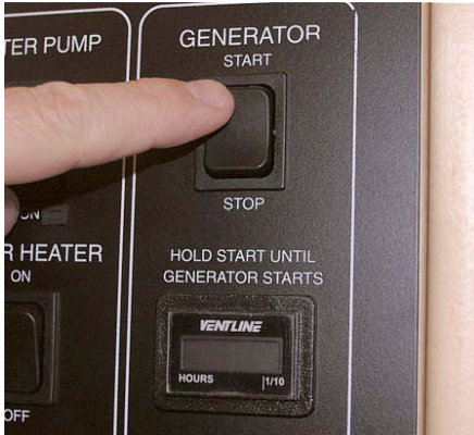
Generator Switch and Hourmeter on Monitor Panel
