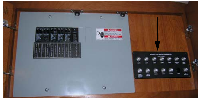
House 12-Volt Circuit Breaker Panel
