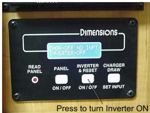
Inverter/Charger Control Panel
