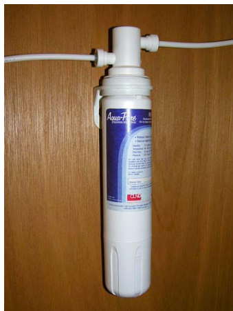
Water Filter Assembly below Galley Sink
