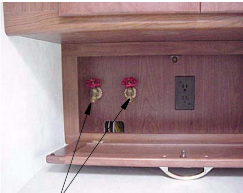
Water Supply Faucets - Typical
