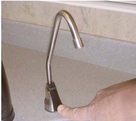
Filtered Water Faucet
