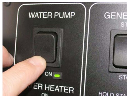
Water Pump Switch
