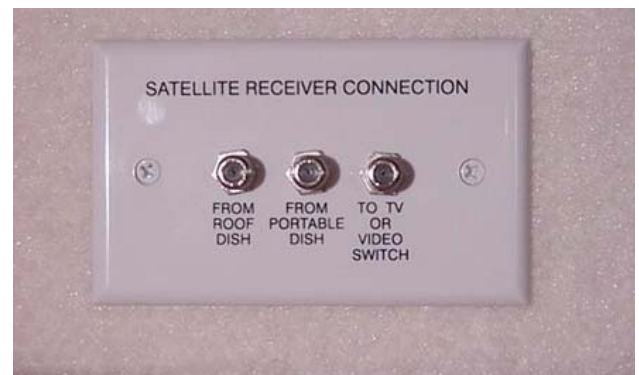
Interior Connection for Satellite Dishes (Located in cabinet near TV) - Typical View
