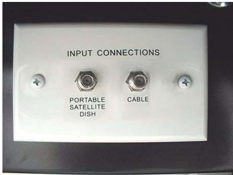
Exterior Connection for Satellite Dish and Cable TV (In Utility Compartment)
