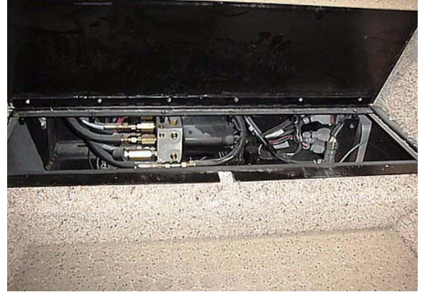
Hydraulic Pump (Beneath entrance step) - Typical View
