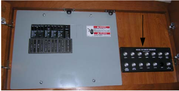
House 12-Volt Circuit Breaker Panel
