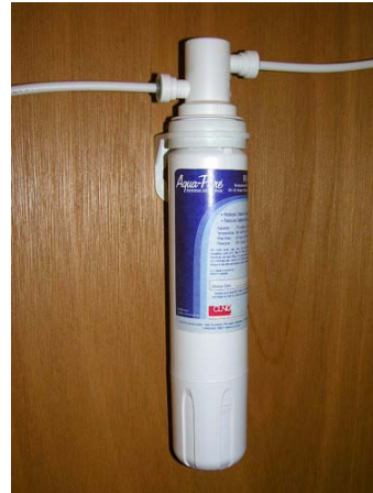
Water Filter Assembly below Galley Sink
