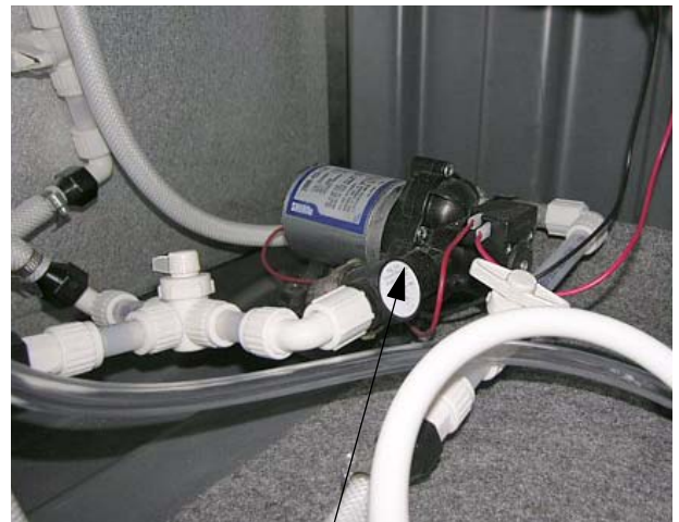
Water Pump (Typical)
